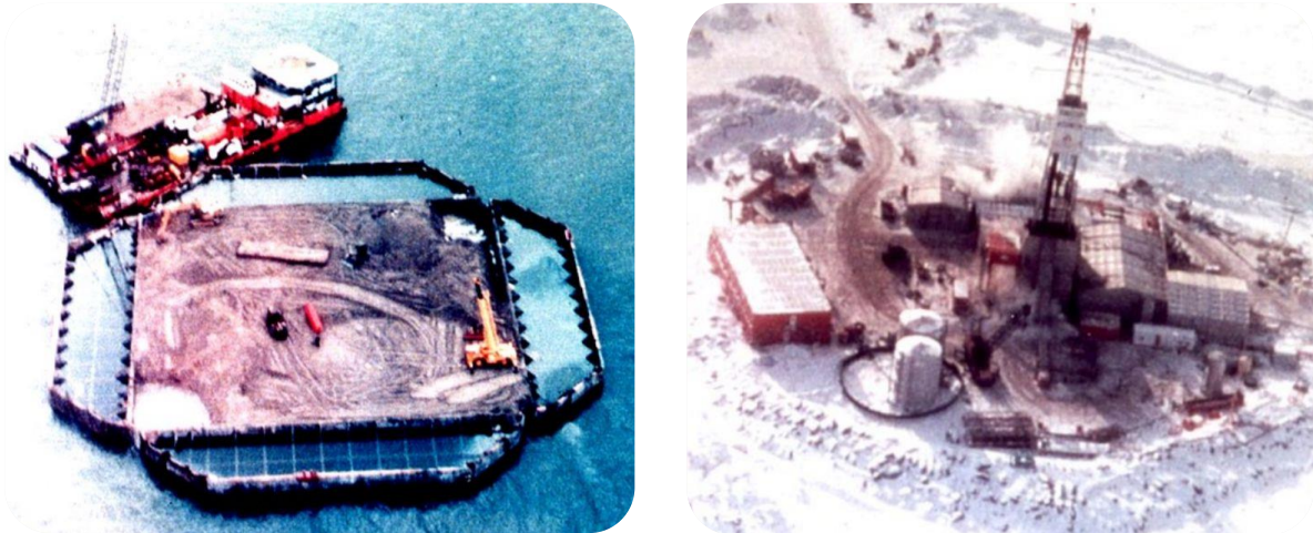
Figure 5.17 Caisson-retained island Tarsuit at different stages. Ballasted ring caisson and beginning of dredged sand infill (left) and completed island with drill in operation under full ice cover (right). From www.bittner-shen.com
